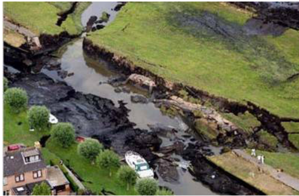
Fig. 1. A levee failure in Wilnis, the Netherlands. This levee breach was caused by the enormous drought in the summer of 2003.
